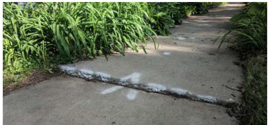
Figure 38: Sidewalk in need of replacement
