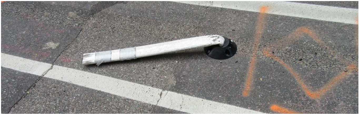
Figure 60: Bollard not maintained
