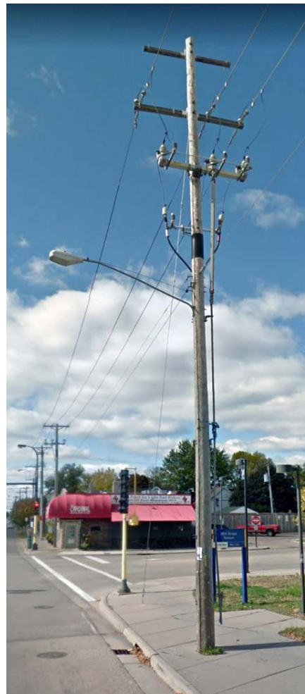
Figure 34: Wood pole streetlight
