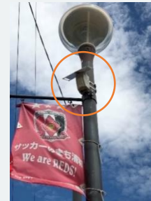
Photo of antenna
