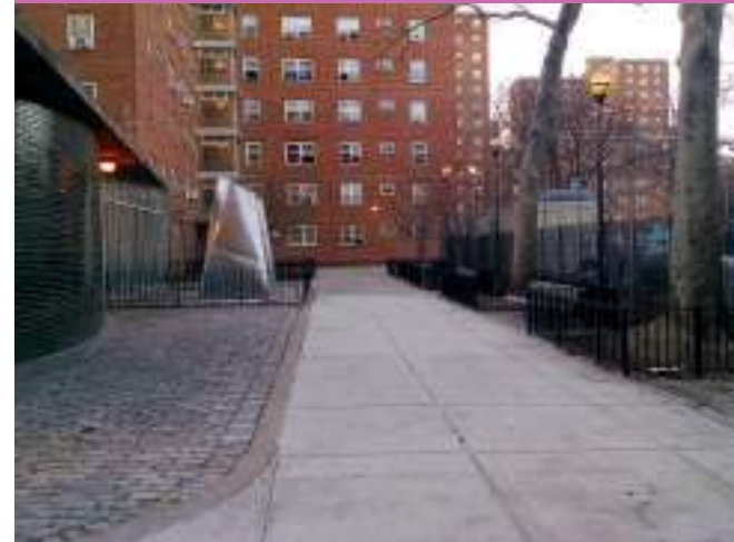
Pathway at Johnson House, made of concrete and Belgian blocks, which are easy to replace.
