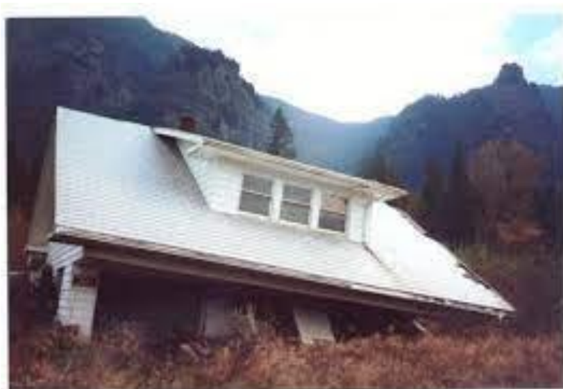
Figure 62 - A home in Dodson, in eastern unincorporated Multnomah County, damaged by landslide in 1996. The house later burned down during the 2017 Eagle Creek Fire.
