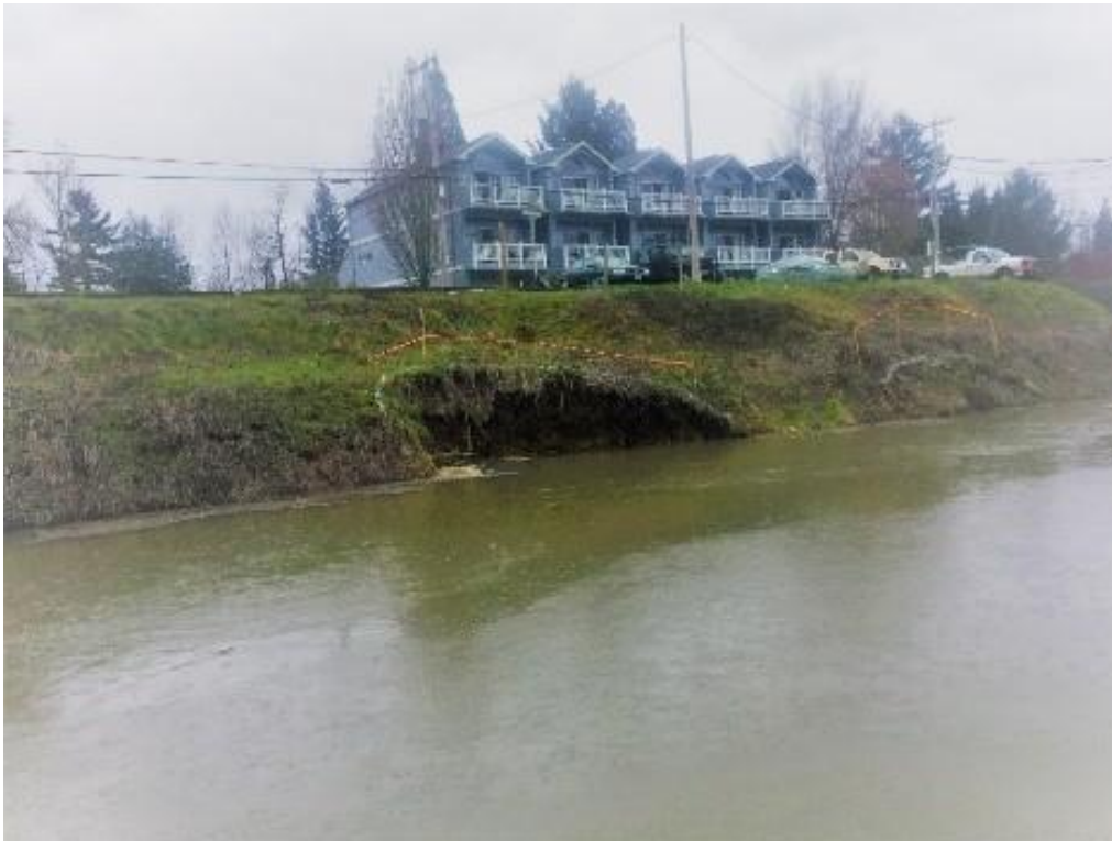
Figure 46 - Levee sloughing damage near NE Bridgeton Rd., in Portland caused by high water during the Spring 2017 flood event. Photo Multnomah County Drainage District.
