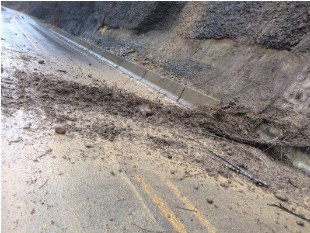
Figure 65 - Minor 2017 winter landslide on the East Historic Columbia River Highway. Photo Multnomah County Sheriff's Office
