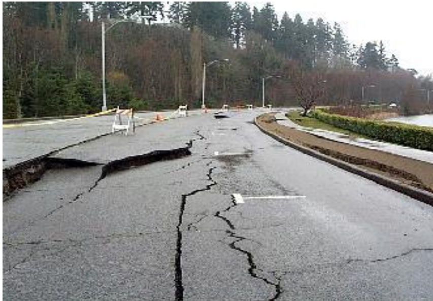
Figure 35 - Road damage caused by lateral spreading in Thurston County, Washington, an impact of the 2001 Nisqually Intraplate Earthquake. Photo – DOGAMI Archive
