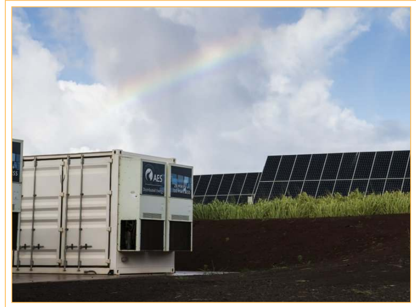
Large solar battery storage hub. Source: US Department of Energy
