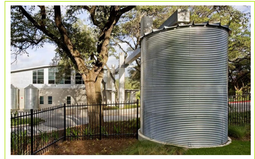
Cistern for water storage. Source: BGK Architects
