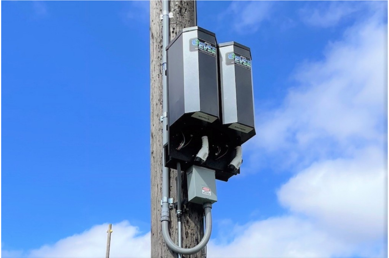
Example of Level 2 EV charger installed on a utility pole
