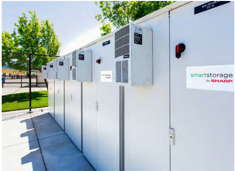
SMART STORAGE SYSTEMS, CALIFORNIA | CREDIT: SHARP
